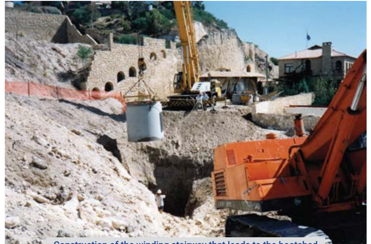
Construction of the winding stairway that leads to the boatshed from Mimi's basement
