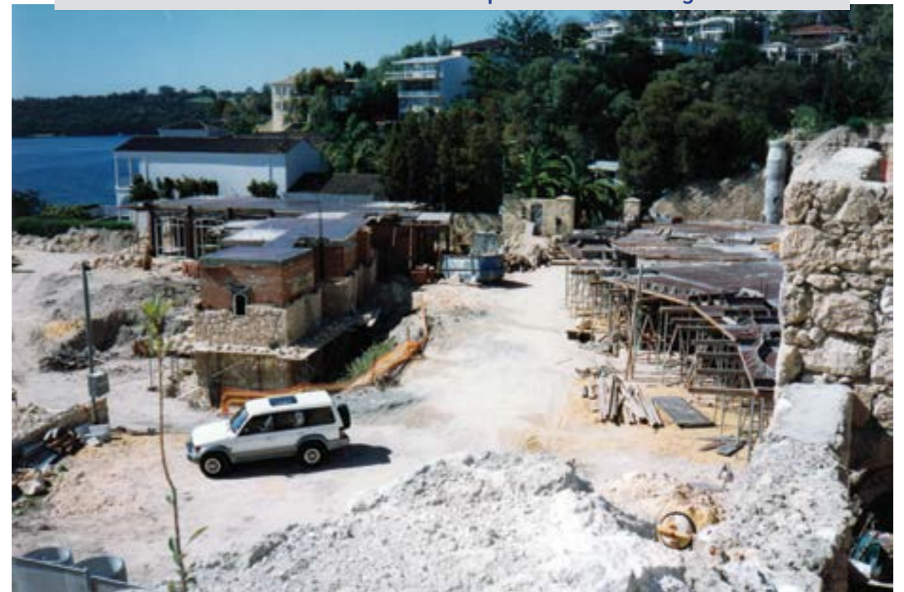
Construction of Mimi's house with the apartments on the right hand side
